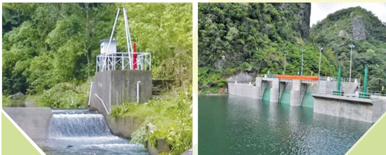
Bukuya Rural Electrification Hydropower project (left), Nadarivatu Hydropower reservoir (right)
