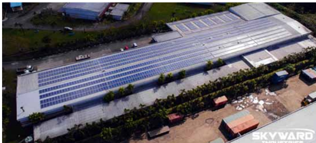
MarkOne Apparel's newly installed solar panels for its Suva based factory, 2014.
