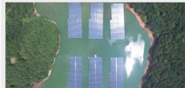
Floating PV in Sang-ju area(6MW)
