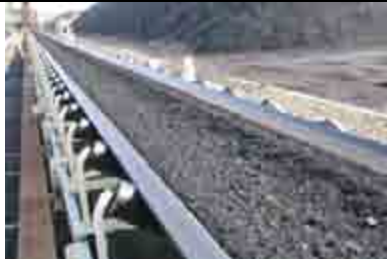
Belt conveyer (receive) 1,550t/h, Length 1.3km
