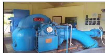
Hydro generation plant
